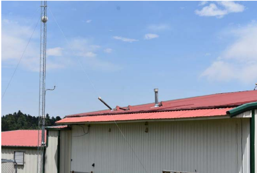
Picture #7.1 – View of the roof, south section. This is a miss-matched culmination of different roofing pitches and as such different flashing. It is recommended this roof section be re-installed and improved.
