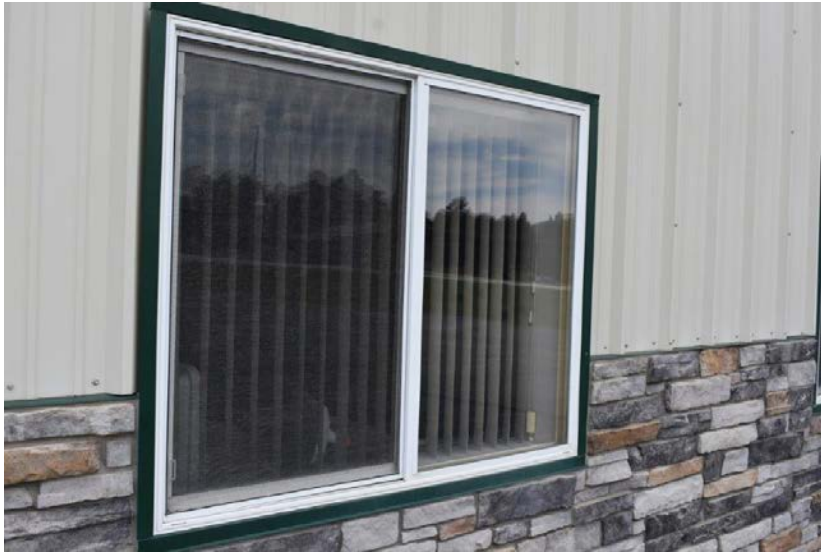
Picture #6.5 – All windows are residential grade, vinyl sliders, in fair condition. It is recommended the windows be upgraded.
