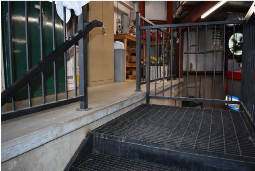
Picture #13.22 – Landing at top of staircase, is not code compliant. Landing should be co-planar with the floor, the current condition creates a hazard.
