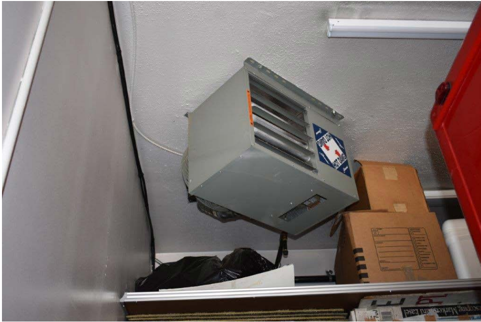
Picture #9.3 – Electric powered convector in the apparatus bay, very energy inefficient recommend replacement.
