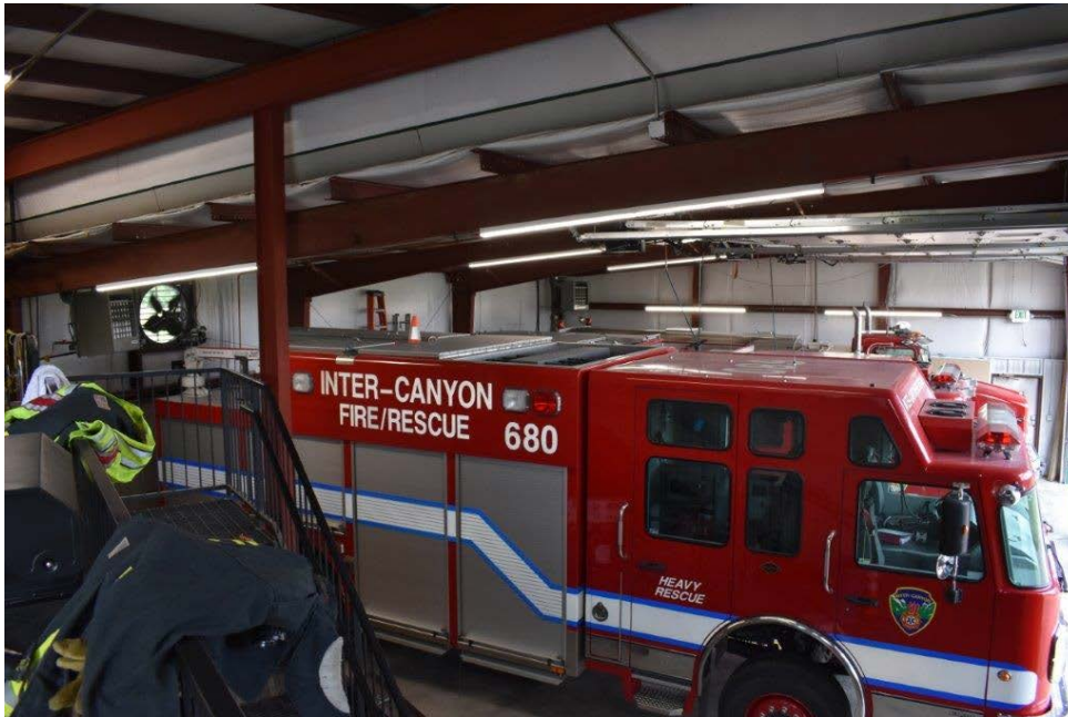
Picture #12.8 – Apparatus bay lighting. Poor lighting for apparatus bay.
