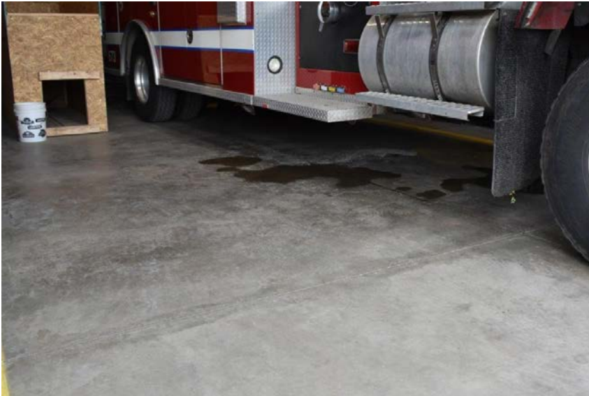
Picture #13.23 – Facility lacks proper floor drains. Standing water creates slip and fall concerns, a safety hazard.
