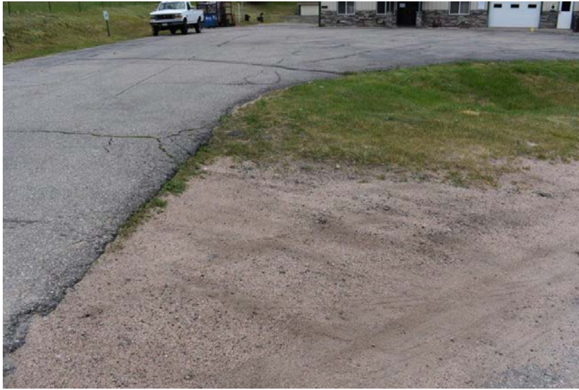
Picture #4.3 – Numerous areas of deteriorated asphalt and areas that should be asphalted.
