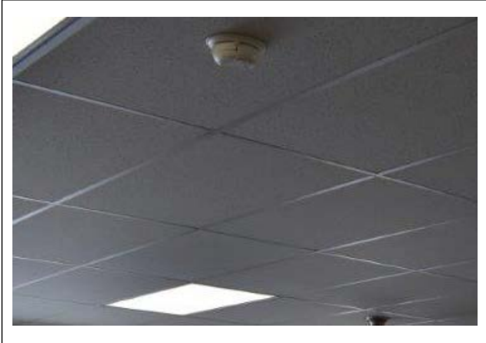
Picture #10.3 – There are smoke alarms in the administration area. Note the dormitory rooms are not properly protected in terms of fire/smoke/CO alarms.
