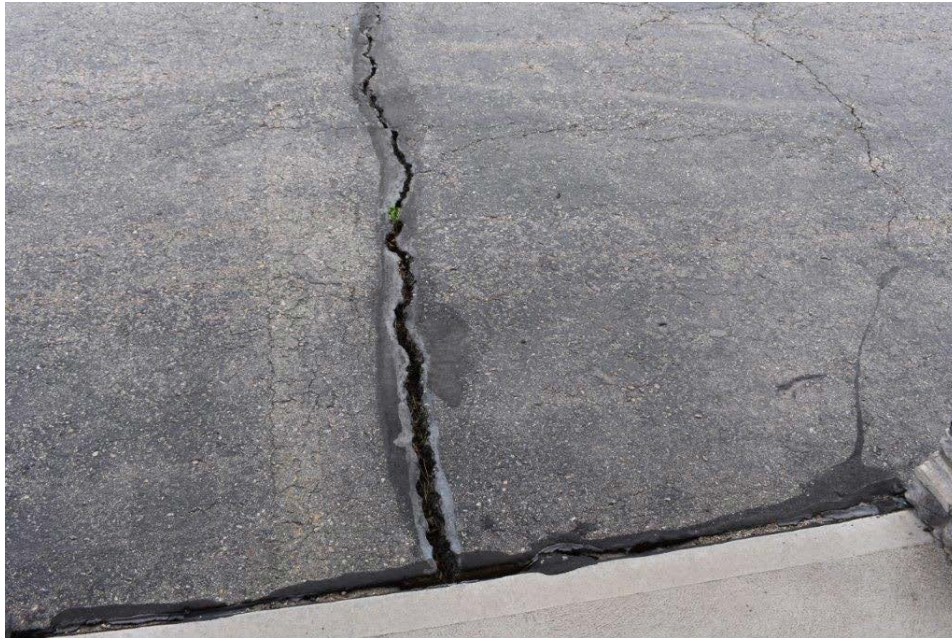
Picture #4.7 – Severe asphalt cracking. These cracks allow water to infiltrate into the subbase beneath and caused more deterioration of the asphalt.
