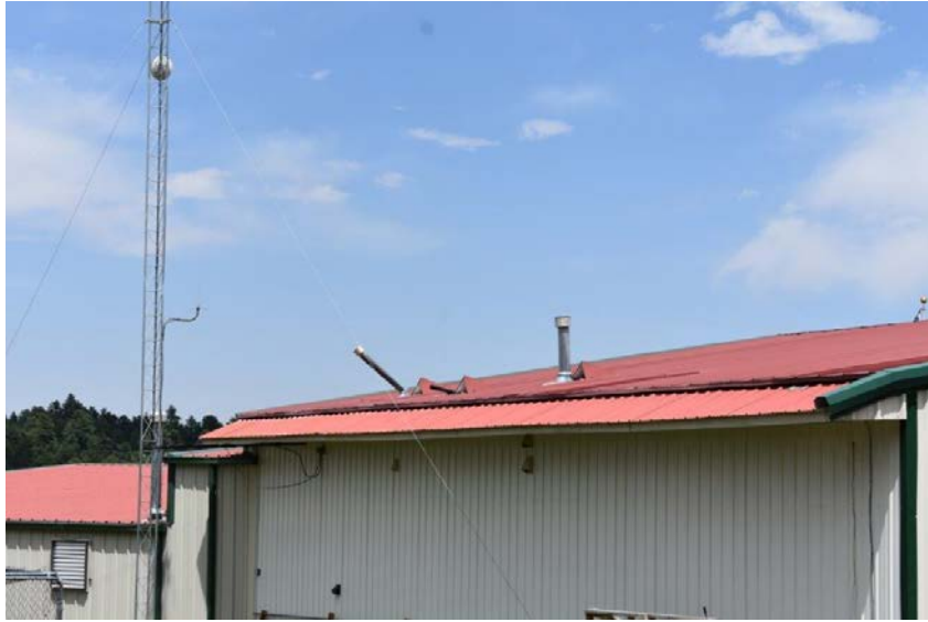
Picture #9.5 – One major concern is the venting of the water heater and furnace in the admin wing. These vents need to be vertical. This could cause an indoor air quality concern and a life-safety issue.
