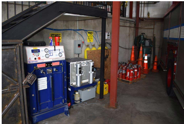
Picture #13.19 – SCBA equipment, improper placement of equipment. Items should all be properly stored and secured.
