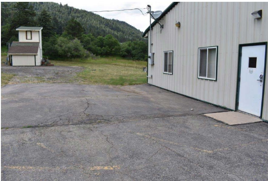
Picture #4.8 – More severely deteriorated asphalt. This area also has poor drainage. Gradient is back to the building which is a problem.
