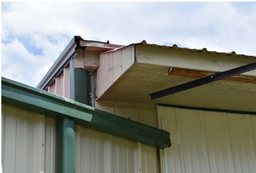
Picture #6.2 – Areas of the exterior envelope, south section are exposed wood in poor condition and poor flashing details. It is recommended this overhang be removed.
