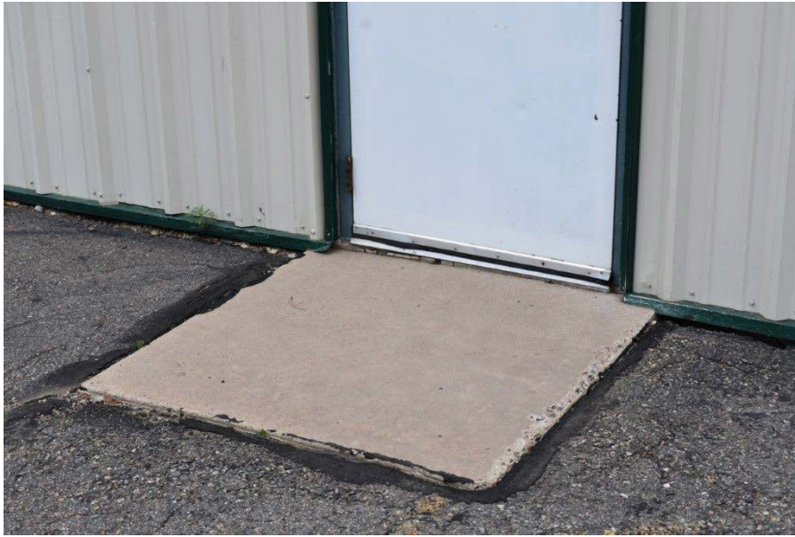
Picture #4.9 – Concrete entrance pad, south door, concrete in poor condition, also the elevation between the concrete and asphalt causes a trip hazard.
