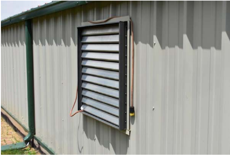
Picture #12.5 – Improper use of an extension cord, life-safety hazard.
