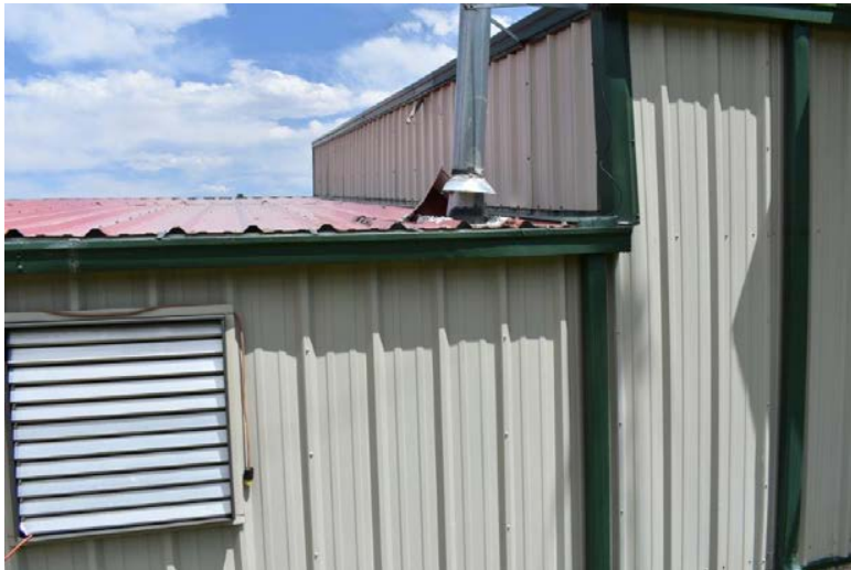
Picture #7.2 – Flashing around the vent stakes is poor and needs to be properly flashed.
