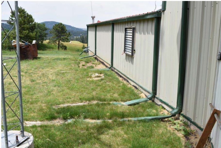
Picture #4.12 – Roof drainage system is damaged, allowing stormwater to collect at base of the building.
