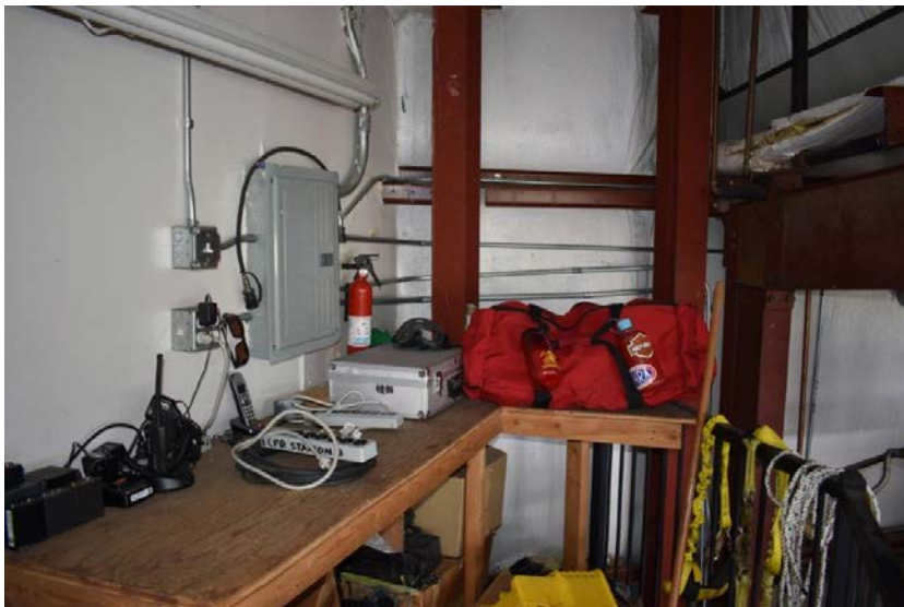
Picture #12.4 – Sub-panel, proper clear space is not provided. This is a code violation.
