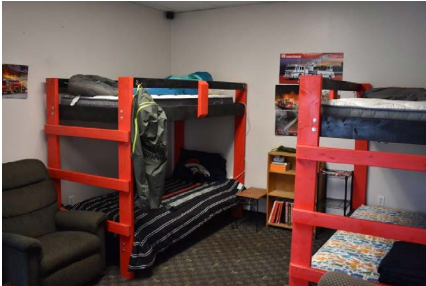
Picture #13.10 – The facility provides only one “crew bunk room”. Separate bunk rooms are required for men and women. Also the room is not code in terms of fire separation requirements and exits directly to the apparatus bay, causing a health hazard.
