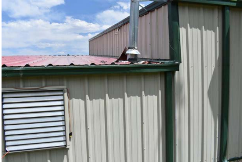
Picture #6.1 – Envelope detail, siding is in fair condition, but there are areas subject to weather infiltration.
