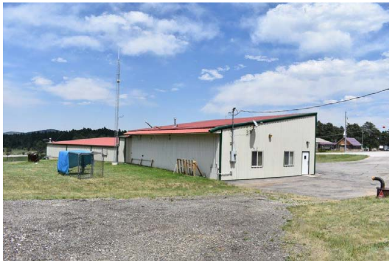
Picture #12.2 – Entrance point of electrical service.
