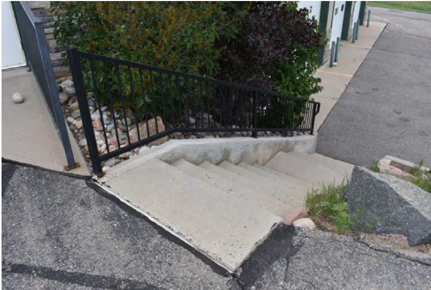
Picture #4.5 – Exterior concrete steps, are non-code compliance and concrete is in poor condition.
