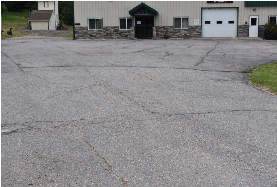
Picture #4.2 – Asphalt is in poor condition. Numerous areas of cracking, alligatoring, and in overall poor condition.
