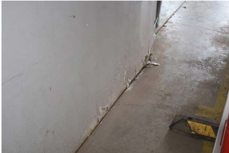
Picture #13.12 – Numerous areas of damaged drywall. This could be a prelude to mold concerns and possible indoor air quality concerns.
