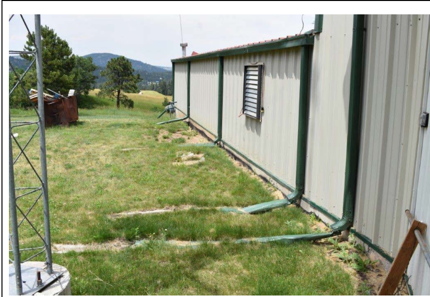
Picture #7.3 – The roof drainage system is deteriorated, damaged, and needs replacement. This is causing improper roof drainage and conveyance problems.
