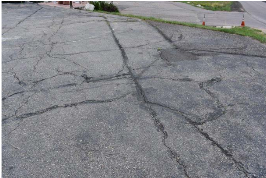
Picture #4.4 – Evidence of poor asphalt.
