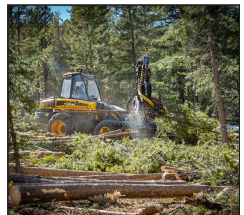
Large equipment will be used to remove trees up to 28 inches in diameter.
